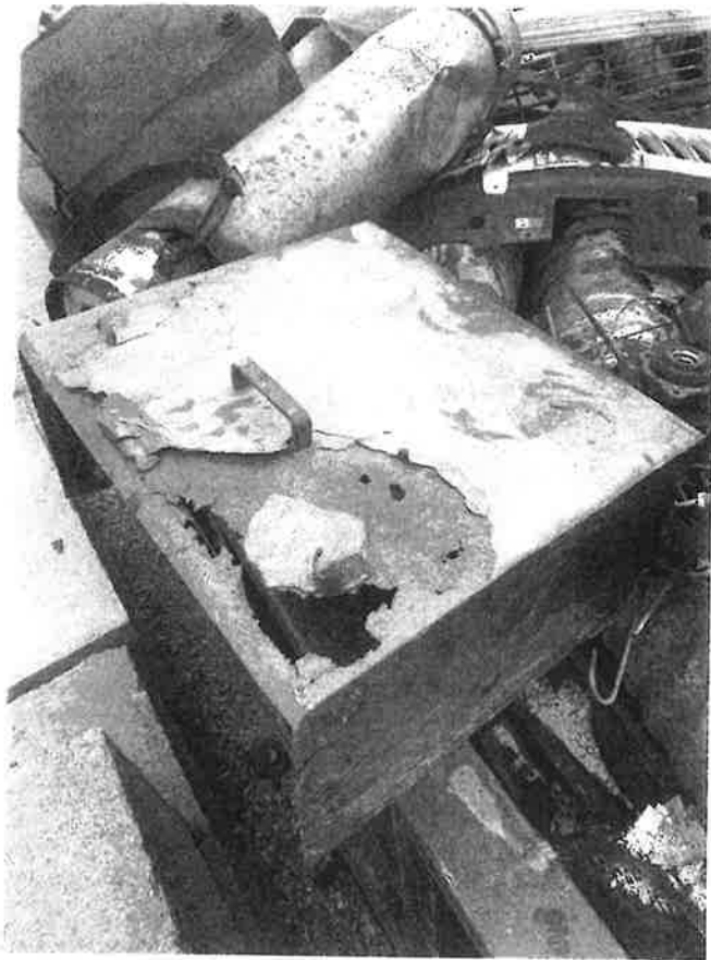
Hydraulic controls cover
